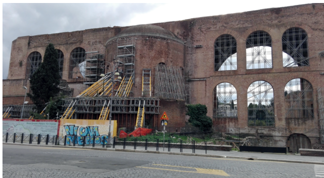
Figure 4.2. Reinforcement of Basilica of Emperor Massenzio along via dei Fori Imperiali during the construction of metro C in Rome, © L. Migliorati.
