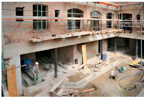
(a) Removal of a supporting wall to open the basement spaces to the interior of the existing atrium
