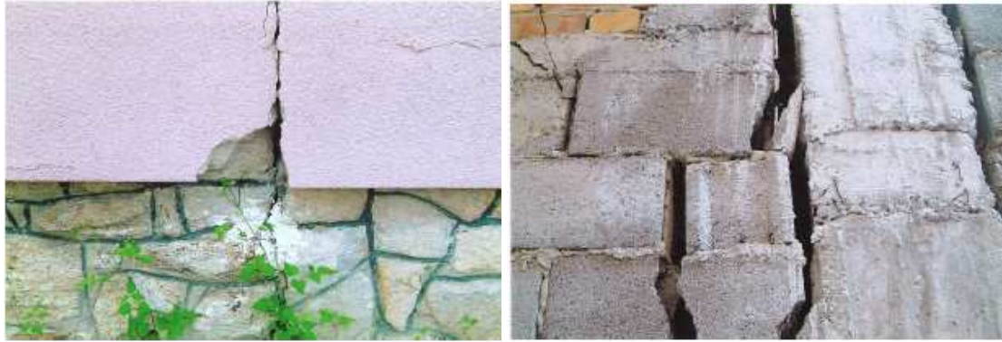
Figure 5: a) Donja Planina 13- south facade – cracks with horizontal right movement with size 3cm [7]; b) A brand new unfinished house in Gornja Planina is located on the fault in the fault zone Stubica - Kašina. Visible movement on bricks, size of 2-3 cm.
