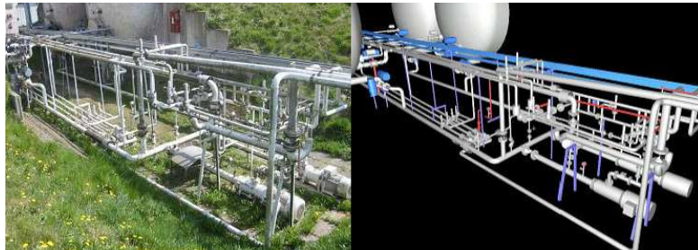
Figure 6: Pipeline of liquid propane in the company Boie in Lübeck
