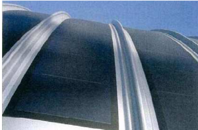
Figure 7. Framed panels with integrated thin-film modules
