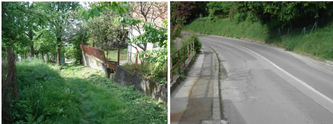
Figure 3. a) In Gornji Mikulići on the route of main fault of the Zagreb zone the landslide has been reactivated in 2008. b) Particularly noticeable are shifts of the ground north of the road, where considerable damage to fences has been recorded [7].
