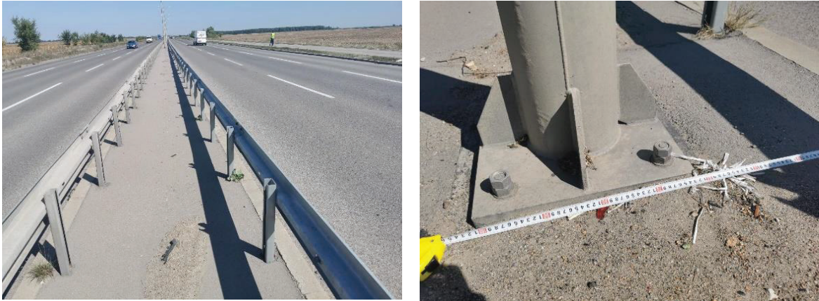
Figure 6. Inadequate median width
