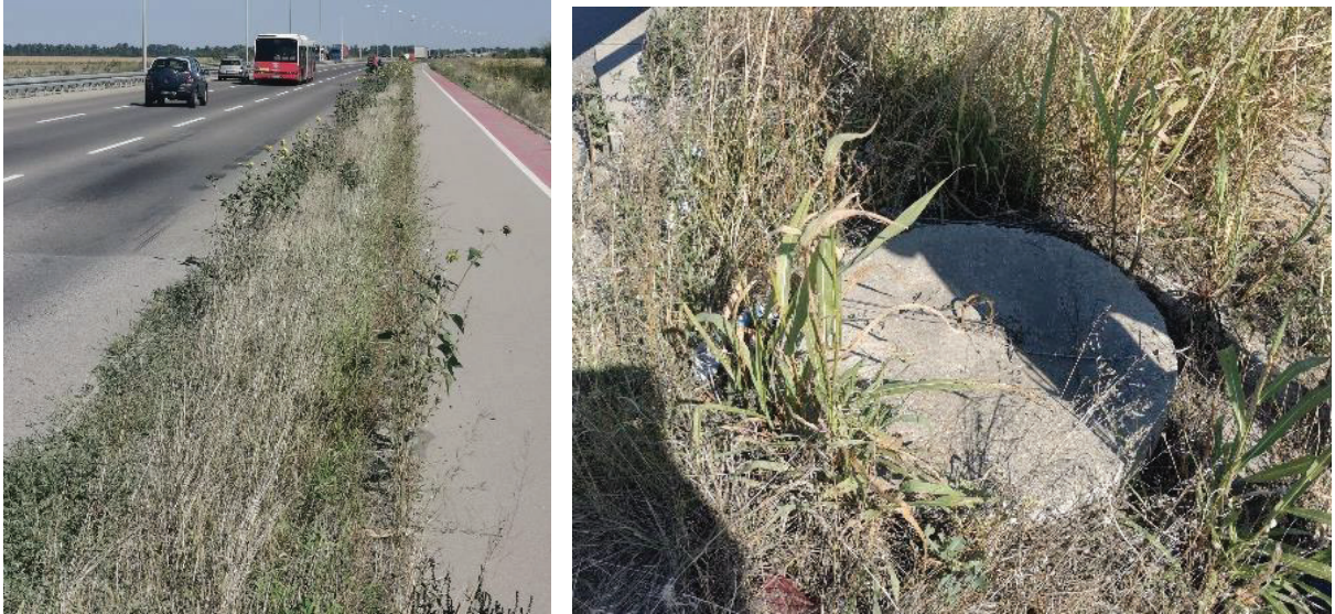
Figure 9. Poorly maintained green belt and drainage system
