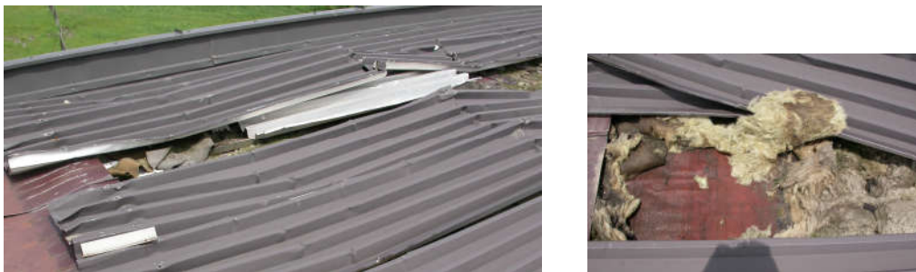
Figure 2: Roof cladding damages.
