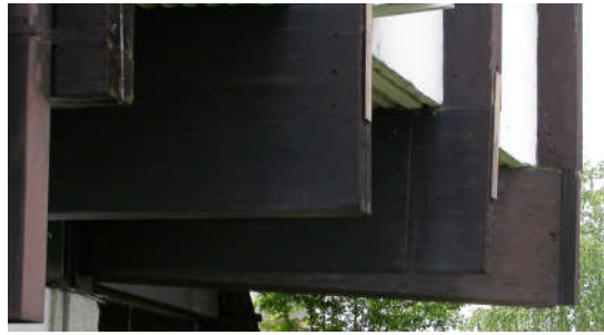
Figure 5: Deflection of the floor beams overhangs.
