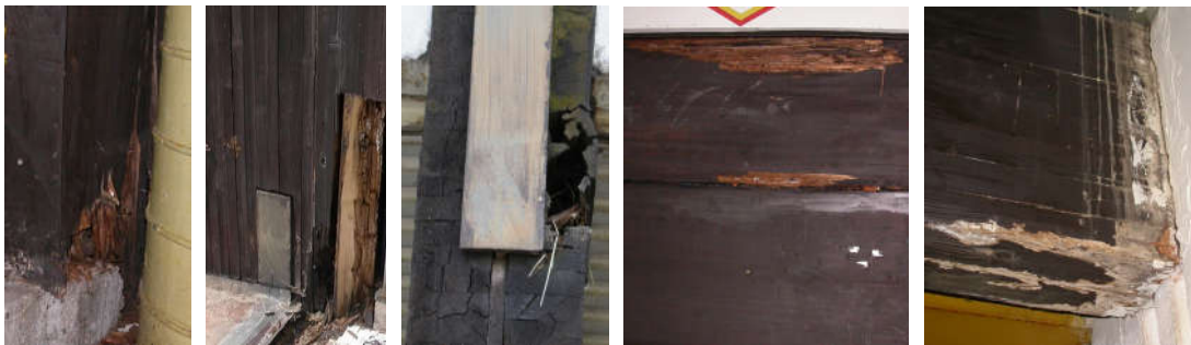
Figure 3: Rotting of timber elements.
