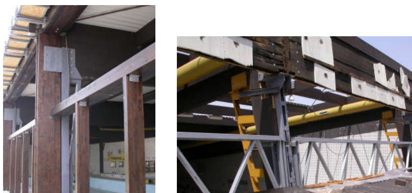
Figure 10: Elements of the new glass facade structure in Z axis (left) and F axis (right).
