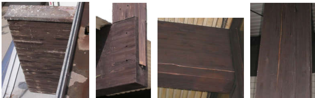
Figure 4: Appearance of fractures and cracks in timber elements.
