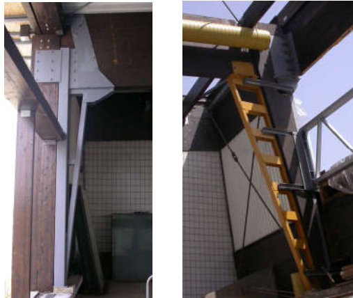
Figure 9: New steel columns next to the existing timber columns in Z axis (left) and F axis (right).
