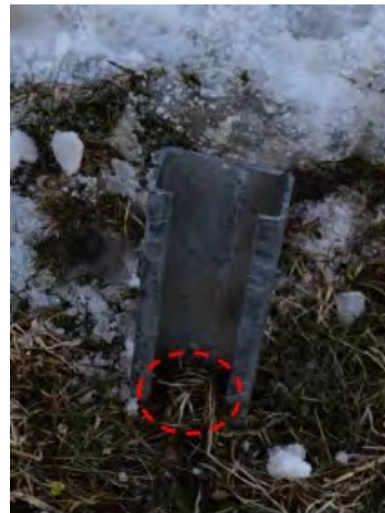
Figure 7: The appearance of the anchor POS 1 after testing
