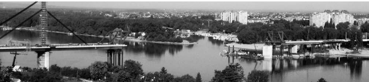
Fig. 18 The "Sloboda" roadway bridge over the River Danube in Novi Sad - under reconstruction
