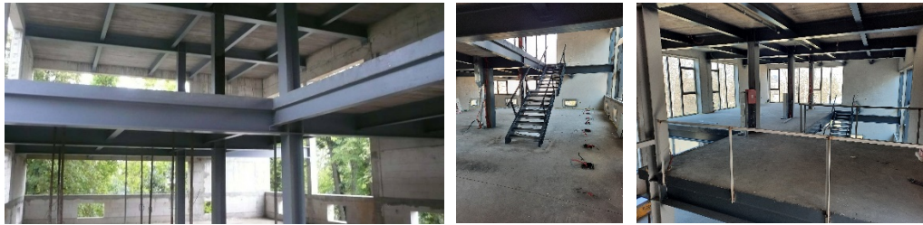
Figure 4. Steel construction of the upgraded part of the building / future library (Photo by author)
