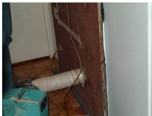
Figure 7. Outside of prefabricated door connecting measured pipe and fan
