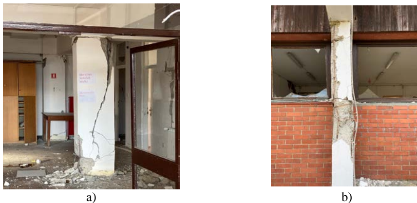
Figure 5 – Damage in the former elementary school in Donja Bačuga: a) shear failure of an interior column and b) a “short column” failure of an exterior column
