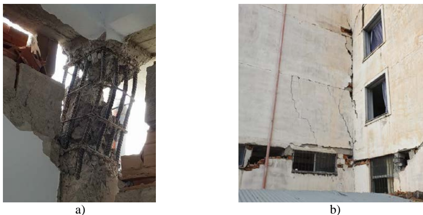
Figure 2 – Damage of a school building in Maminas, Albania: a) failure of the RC column and b) damaged masonry infill walls [6]
