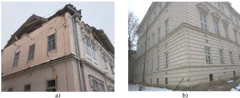
Figure 3 – Damage of URM schools in Petrinja, Croatia: a) exterior damage of the First school building and b) inclined shear cracks in the walls of the Petrinja High School
