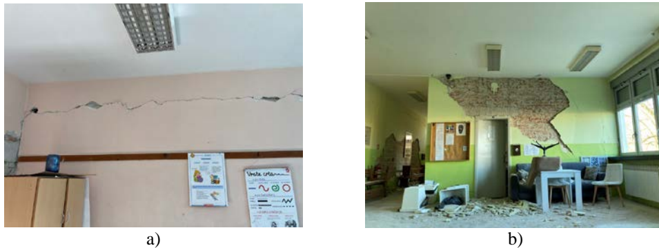
Figure 4 – Damage of RC schools in Petrinja, Croatia: a) cracks at the infill-frame interface, school Dragutin Tadijanović and b) damage of infill walls and plaster spalling, the Faculty of Education
