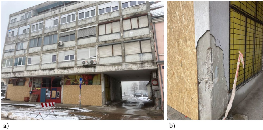
Fig. 33 Damage of type RC1 residential building in Petrinja, Croatia due to the December 2020 earthquake: a exterior view showing open ground floor space which used as a store before the earthquake, and b a detail of the damaged RC column (SUZI-SAAE 2021)
