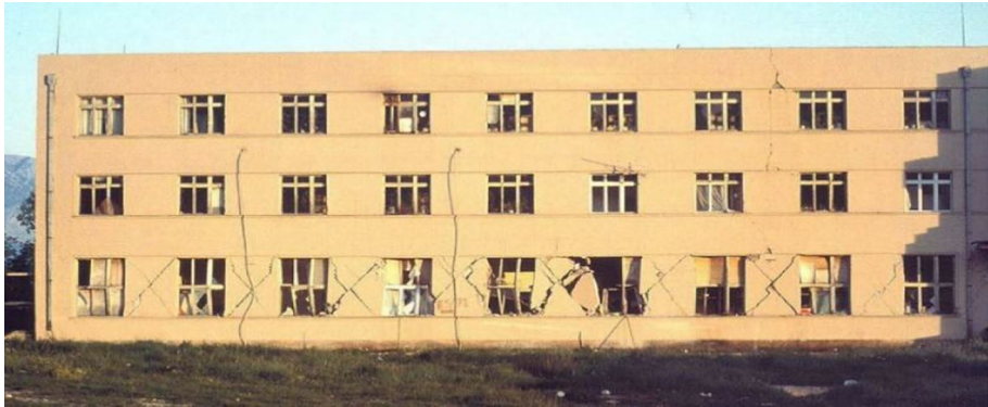
Fig. 25 Budva Town Hall—an example of a type M3-M building damaged in the 1979 Montenegro earthquake (M. Fischinger)
