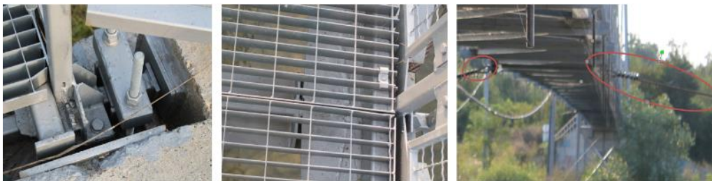
Figure 8. Characteristic details of the footbridge – deck end supports, pedestrian walk board and side ropes, respectively
