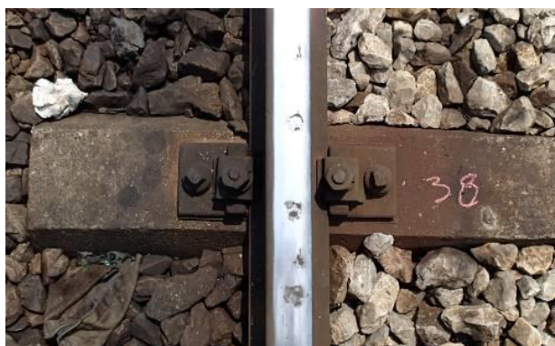
Fig.2. Successive occurrence of squats (left rail, track No. 2, Pančevo Varoš station, 2017)
