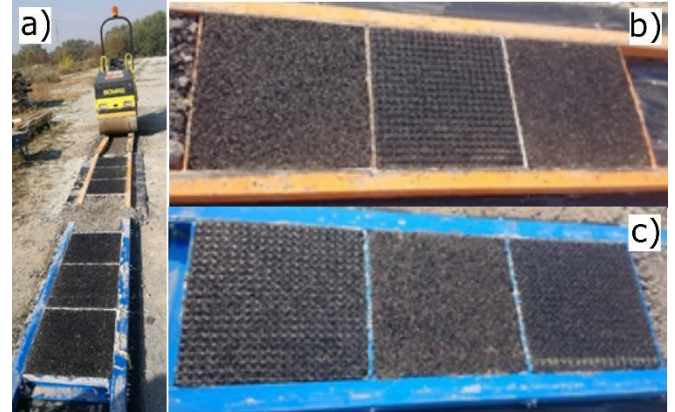
Figure 1. (a) Compaction of slabs with a 1-ton roller and (b, c) compacted bottom layers with and without glasgrid
