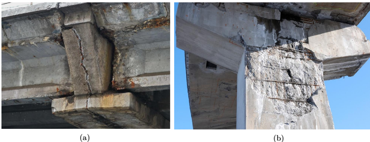
Figure 2.6. Damaged piers: (a) Cracked pier cap, (b) large spalling on the pier.
