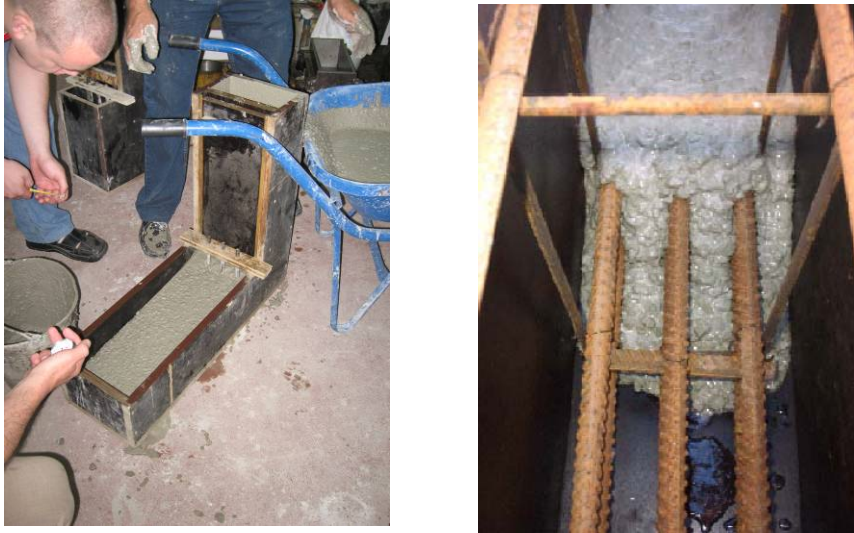
Figure 1. L-box test, commonly used for passing ability assessment of fresh state SCC mixture (left), and an illustration of on-site behavior of SCC (right), covering densely spaced reinforcement bars
