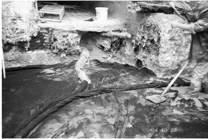
Fig. 4 - Drainage pipe made for thermal spring water
