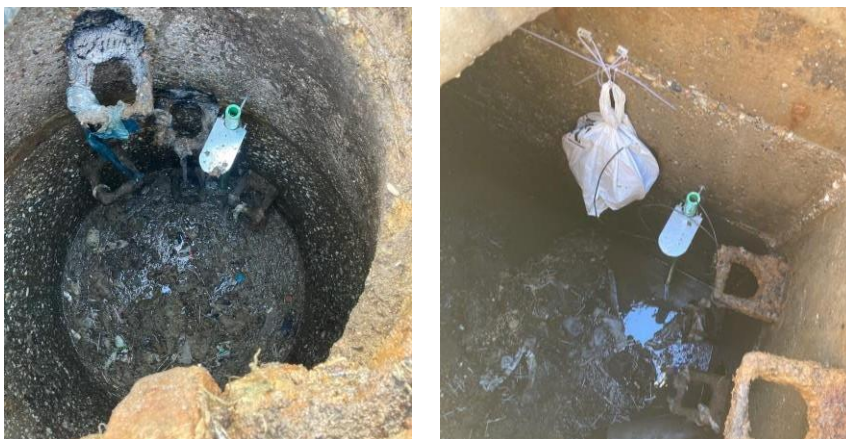
Slika 1. Stanje u Š SP2 i Š SP3 , tokom montaže opreme Figure 2. Manholes Š SP2 and Š SP3 state in regular operation
