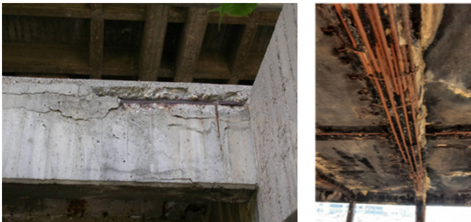
Figure 3 – Spalling of concrete as SLS (left) and ULS (right)
