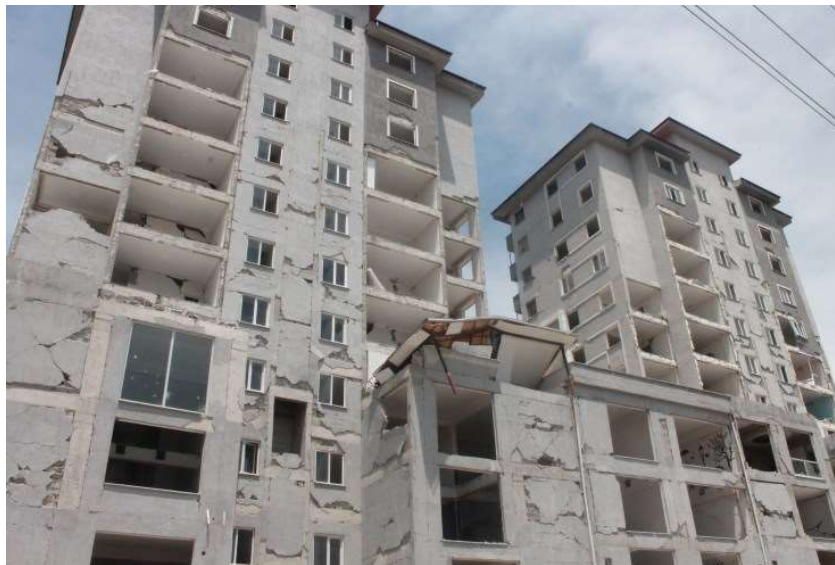
Diagram 11. Failure of exterior masonry infills was observed in all building blocks
