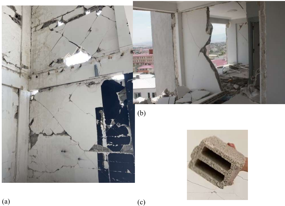
Diagram 12. Non-structural damage of masonry infill walls and partitions; a) extensive cracking of exterior masonry infills and separation from the frame – ground floor level; b) failure of both interior and exterior infills at the upper floors, and c) a typical masonry block.
