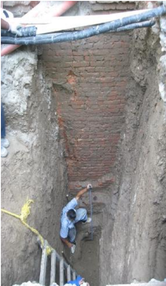
Slika 5. Utvrđivanje dimenzija temelja u jami J-1 Figure 5. Measuring foundation dimensions in trial pit J-1
