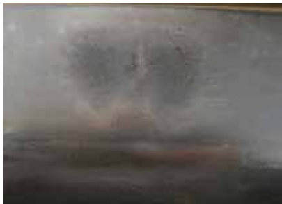
Figure 1. Typical defect in form of "lungs", Vrbnica – Bar Railway, Podgorica – Golubovci Section
