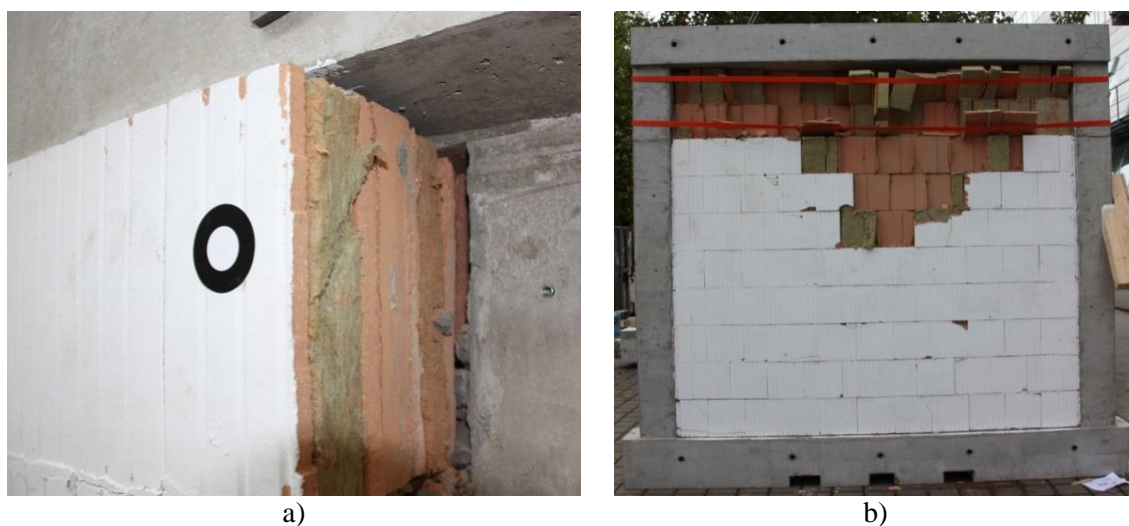
Figure 5.40 a) Failure of the brick in the upper corner of the wall and b) damage of the backside of the wall at the end of the whole loading protocol
