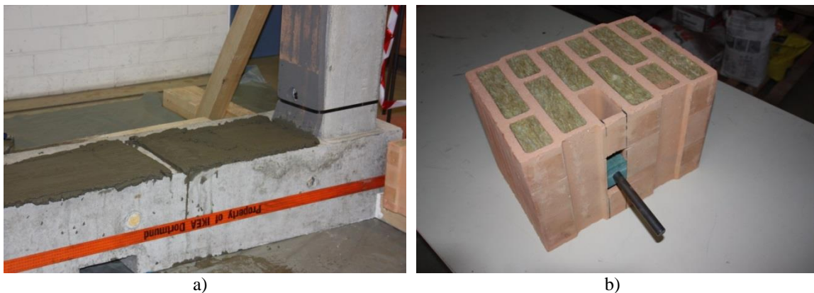
Figure 3.5 a) First layer of normal thick mortar and b) brick with shear anchors and elastomer
