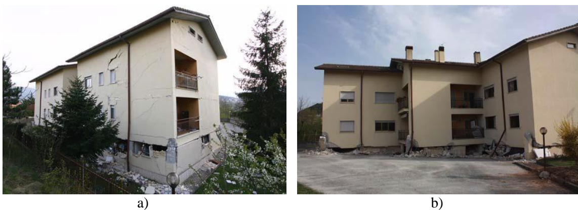
Figure 1.11 Soft storey collapse of a building in 2009 L'Aquila earthquake: a) backside and b) frontside (Dazio et al., 2009)
