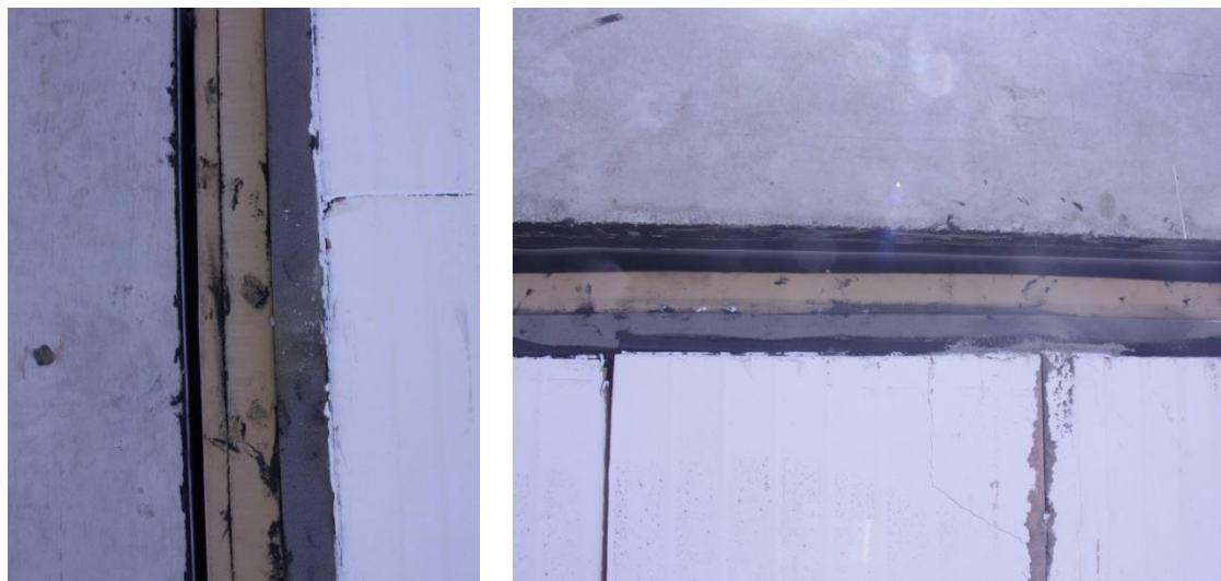
Figure 5.83 Intact glued connection between the U-shaped elastomers and bricks at the end of test
