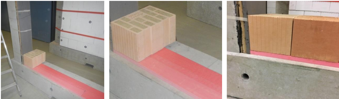
Figure 3.9 Three strips of elastomer at the bottom beam and gluing the first row of bricks on the elastomer
