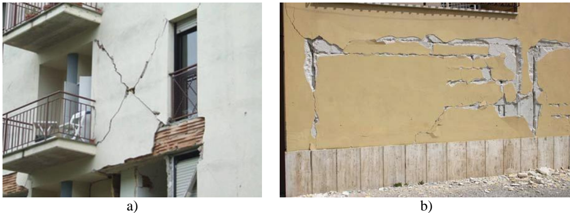
Figure 1.7 a) X cracked infill wall (Braga et al., 2011) and b) horizontal and vertical separation cracks between frame and infill with the horizontal cracks in infill joints (Dazio et al., 2009)
