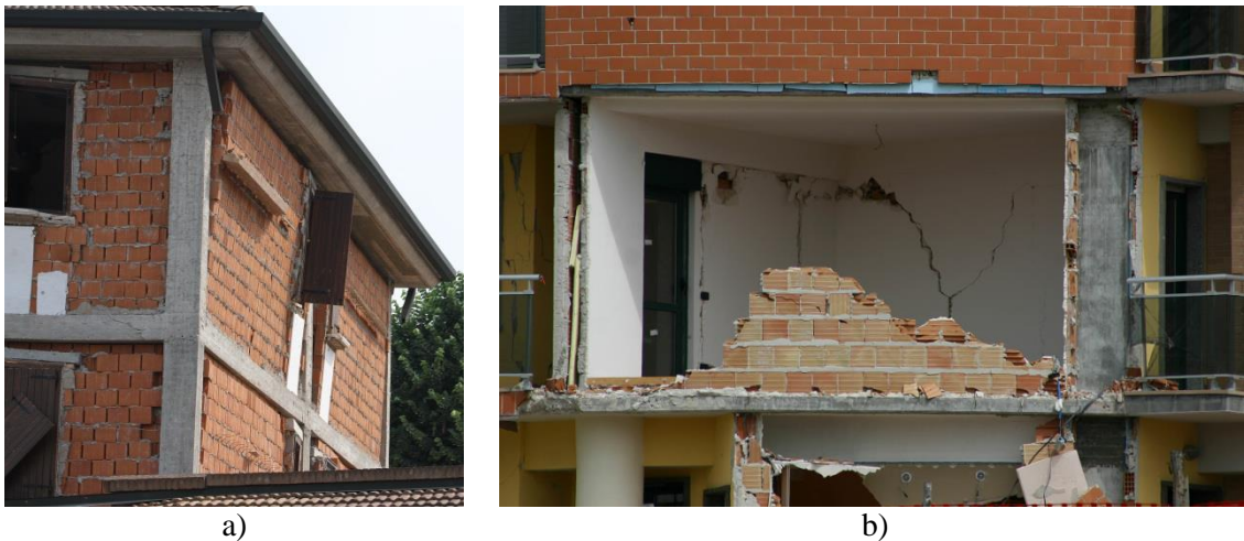
Figure 1.9 a) Damaged infill in Italy: Emilia Romagna (2012) and b) L'Aquila (Dazio et al., 2009)
