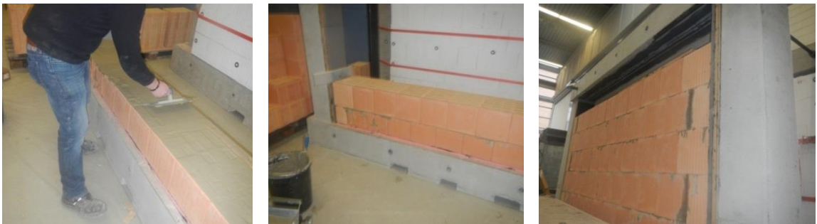
Figure 3.10 Brick up the wall in a usually way but with gluing the edge bricks to the elastomer
