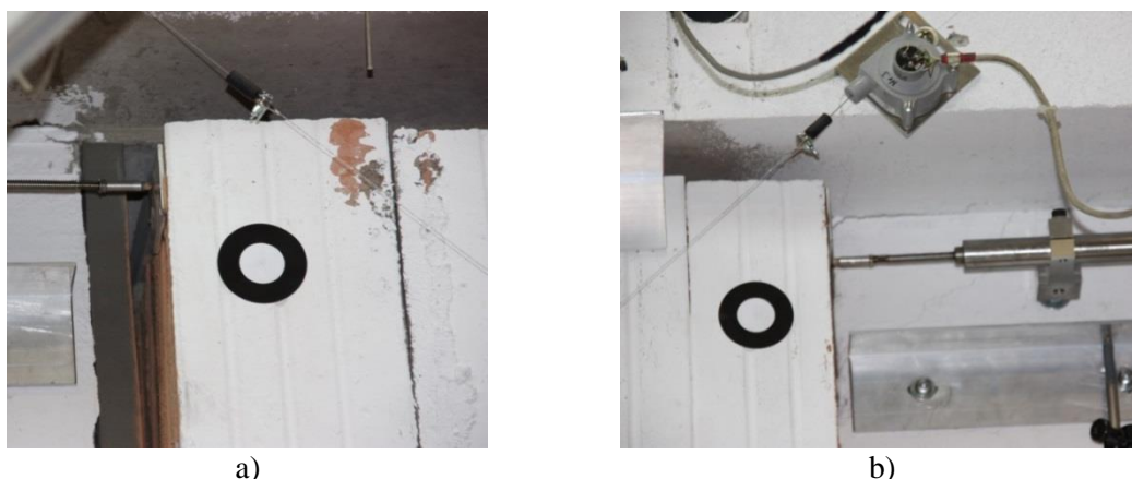
Figure 5.57 a) Gapping and b) highly compressed elastomers at corners
