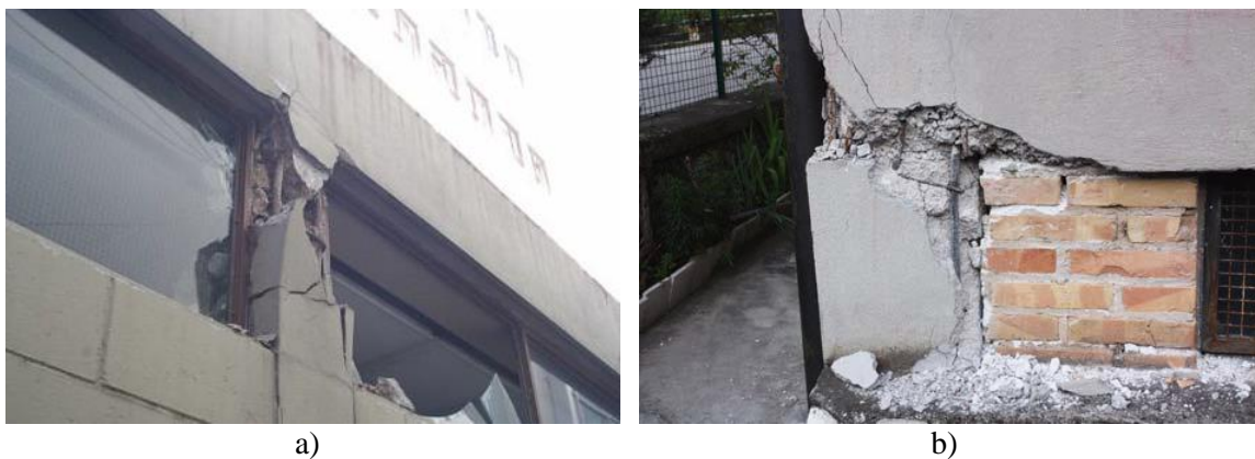
Figure 1.10 a) Short column failure during 2011 Christchurch earthquake (Tasligedik, 2014) and b) 2009 L'Aquila earthquake (Dazio et al., 2009)
