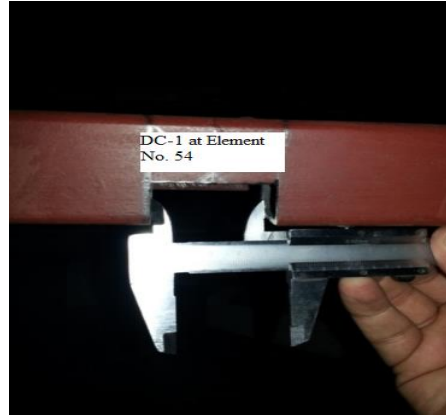
Figure 5.27. Severity of damage scenario in DC-1 on the grid bridge model
