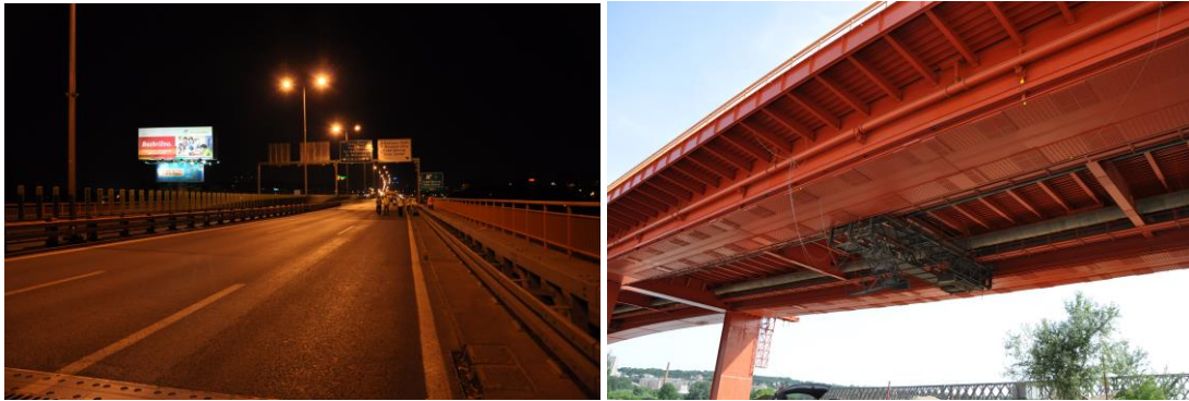
Figure 3.7: Tested GAZELA bridge approach structure on the left bank of Sava river [107]
