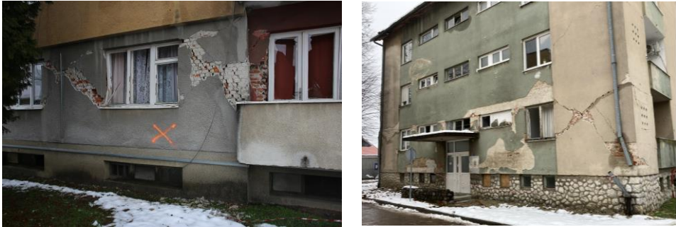
Figure 4. Shear cracking at ground floor level of multi-storey URM apartment buildings in the 2020 Petrinja earthquake
