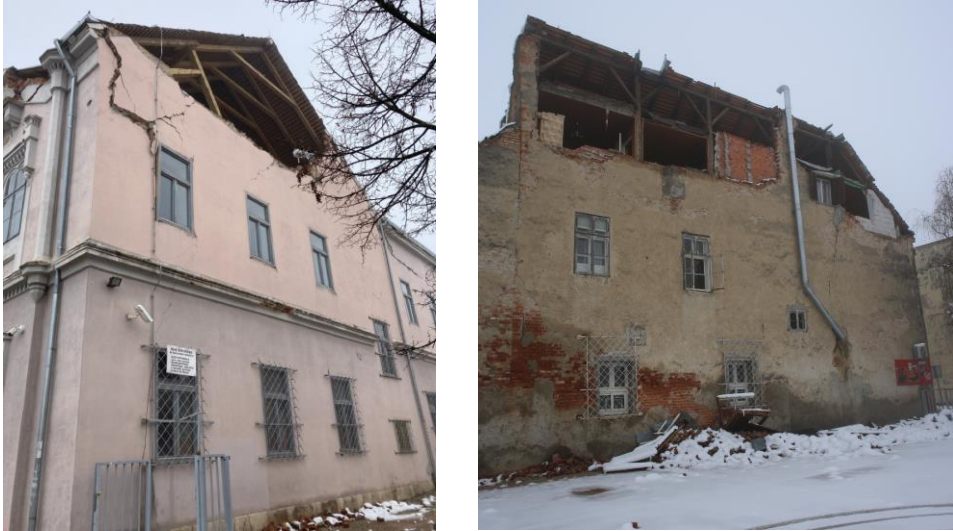
Figure 3. OOP Collapse of URM walls in buildings in Petrinja, Croatia
