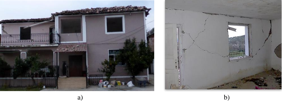
Figure 1. a) Damaged low-rise masonry building made of hollow concrete blocks and b) partial collapse of the demolished building in Thumanë (Albania)
