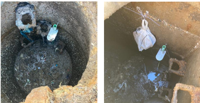
Slika 1. Stanje u Š SP2 i Š SP3 , tokom montaže opreme Figure 2. Manholes Š SP2 and Š SP3 state in regular operation
