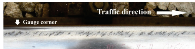
Figure 5 Light HC defect on the straight track section (1 ÷ 4 cracks / 1 cm, length of 5 ÷ 10 mm)
