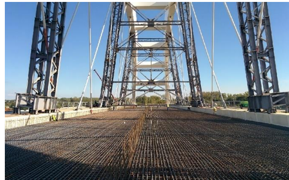
Deck reinforcement installation. The temporary columns for launching are still on place.
