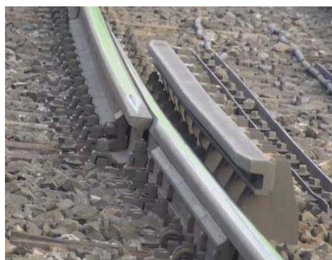
Slika 12. Diskontinuitet vozne površi u zoni dilatacione sprave Figure 12. Discontinuity of the running surface of the rail head at the expansion joint
